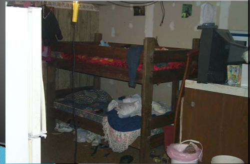
Children's bedroom in basement—no window or smoke detector Using portable light for permanent use
